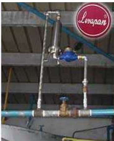
ELCE S1 at Levapan Factory PANAMA
